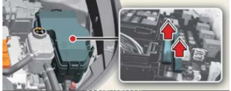
Engine room fuse box
